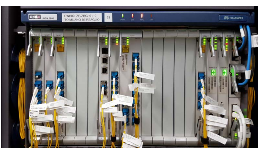
Optical system component by Huawei
