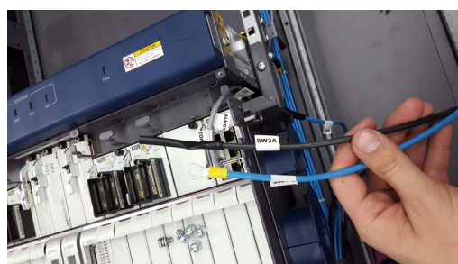
Power connections for Huawei Equipment
