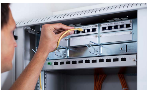
Switchboard with configured rack
